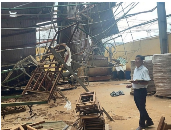
PJICO Binh Dinh carried out claims assessment activities following Typhoon No. 13
